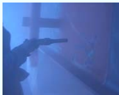
Conventional removal method (causing some scattering of paint coating film dust, noise and odors)
