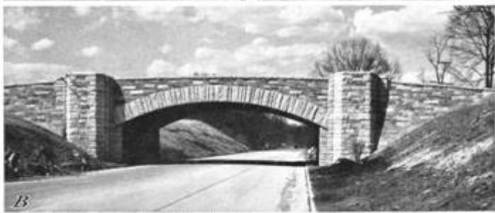
BRIDGES DESIGNED TO BE IN HARMONY WITH LANDSCAPED SURROUNDINGS. GRADING AND LANDSCAPING NOT YET COMPLETED.
