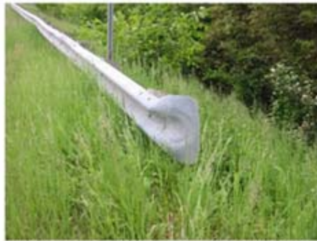
Exposed W-beam spade end
