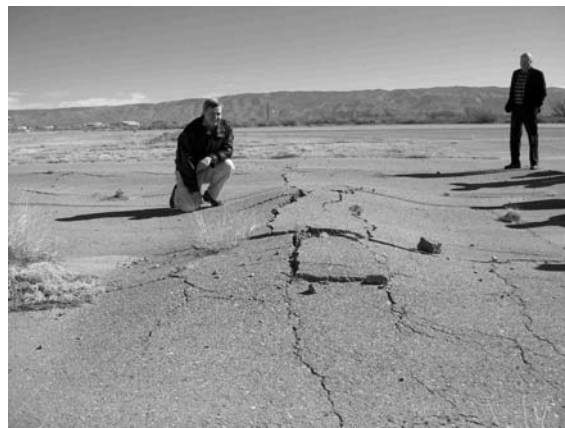
Figure 2 - Swelling caused by sulfate attack on cement-stabilized taxiway base course at Holloman AFB, NM.
