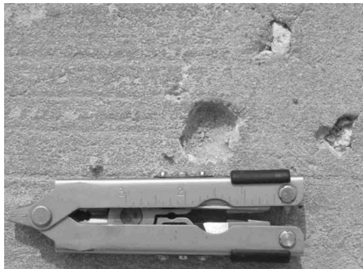
Figure 3 – Popouts from unsound aggregate
