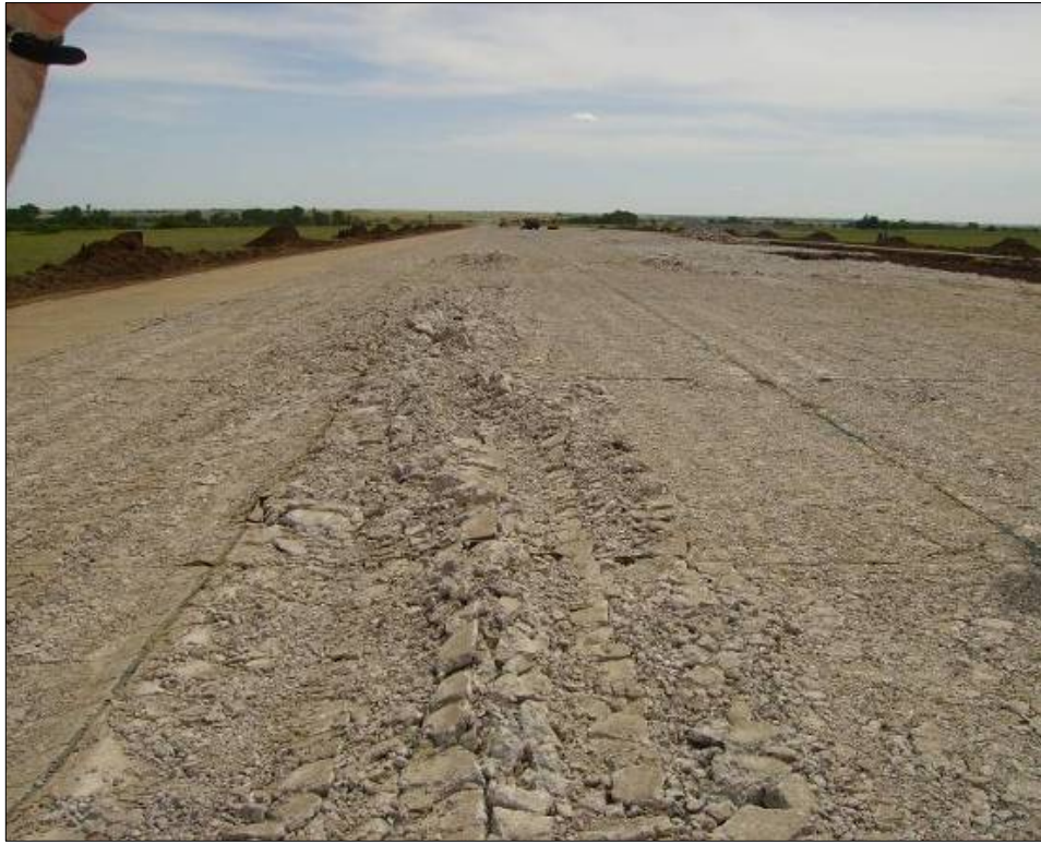
Figure 13. Rutting from RPB of Unstable Area at Kegelman that Requires Excavation
