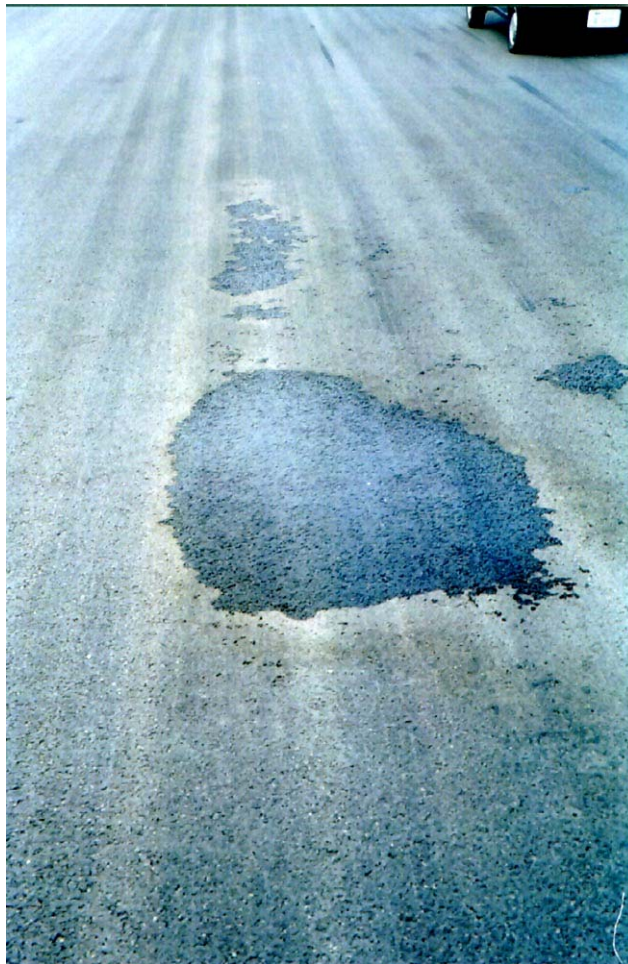
Figure 2 - Water draining up through pavement when inspected in 2000.
