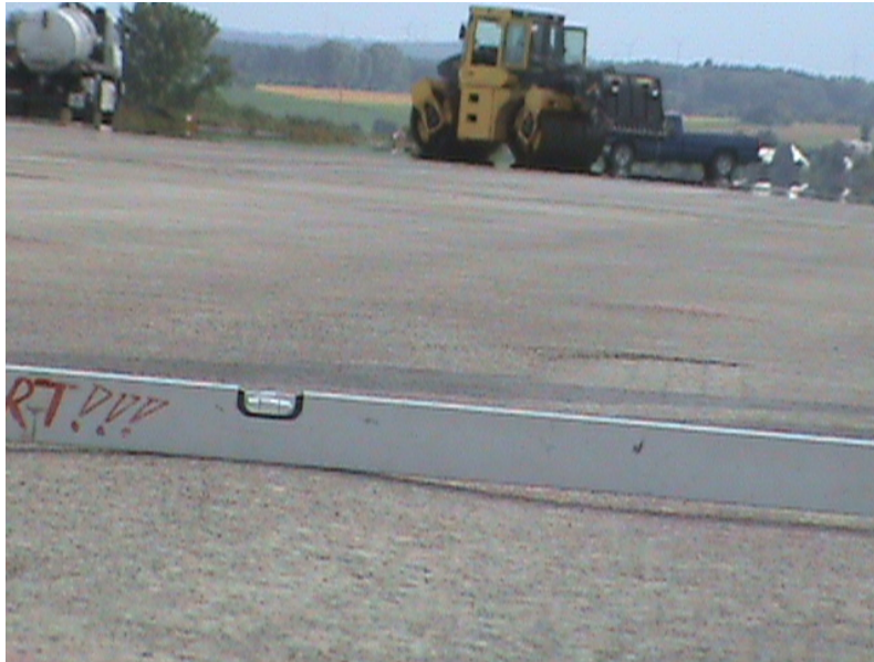
Figure 5 - Blister shown below straightedge.
