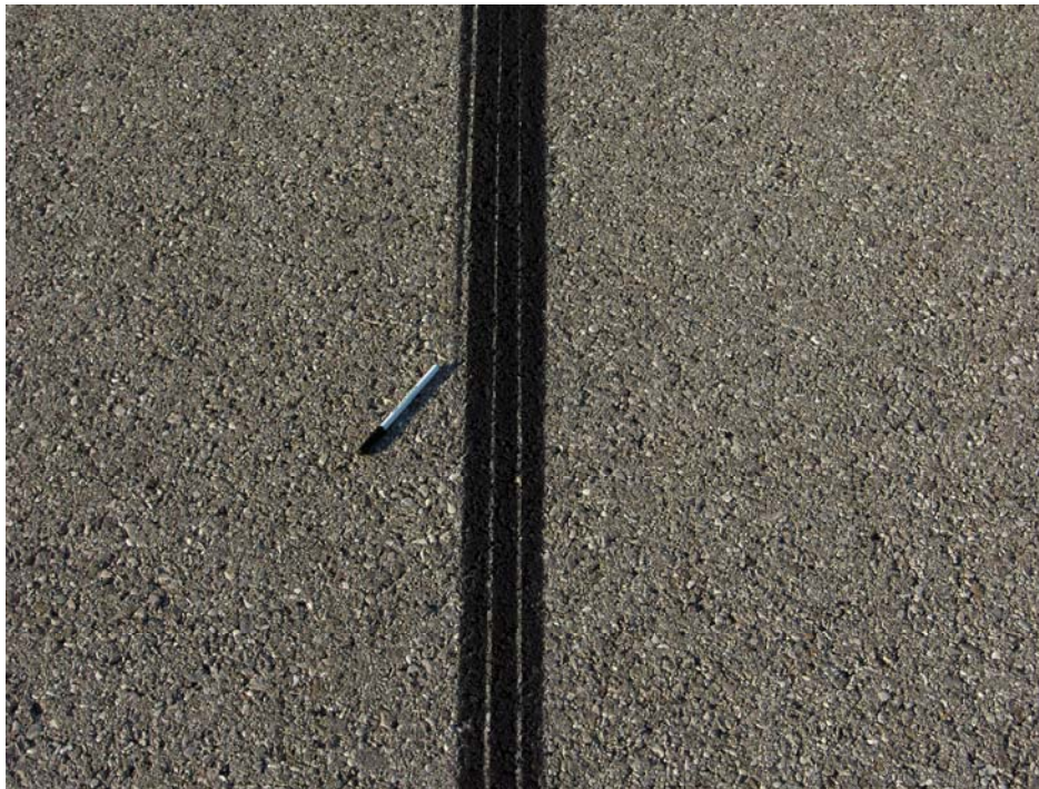
Figure 3 - Condition of SMA Surface with skid mark after 7 years.
