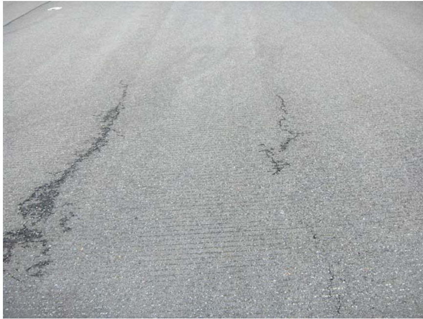
Figure 4 - Cracking with moisture migrating up through cracks.
