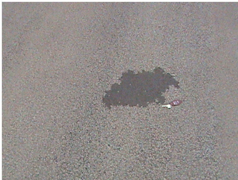
Figure 6 - Water from underlying layers moving through surface in hot weather.
