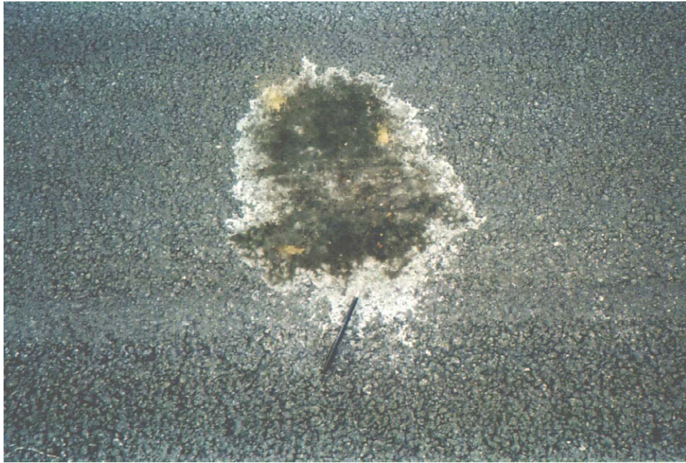
Figure 1 - Fat spot shown during inspection in 2000.
