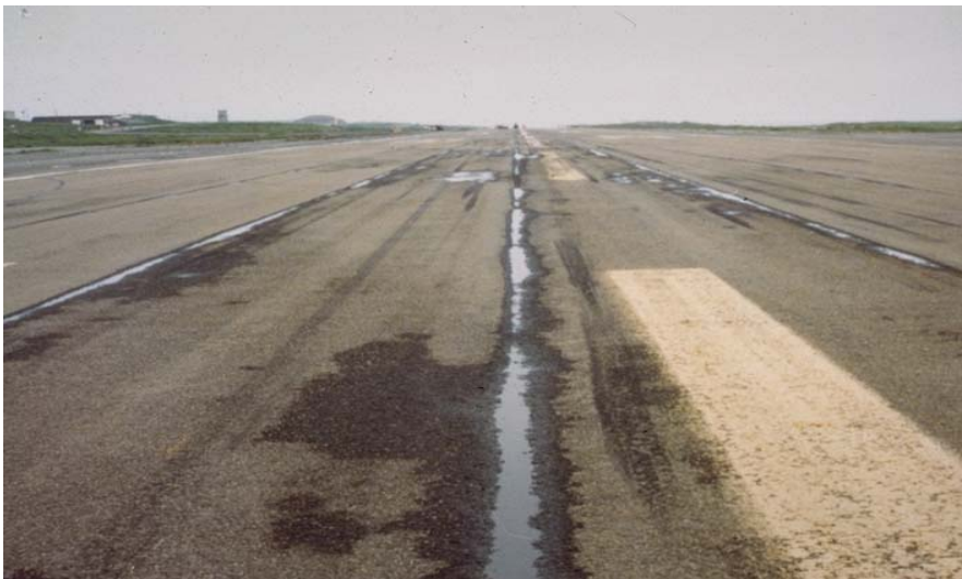
Figure 1. Cracking and Raveling of Longitudinal Joint.
