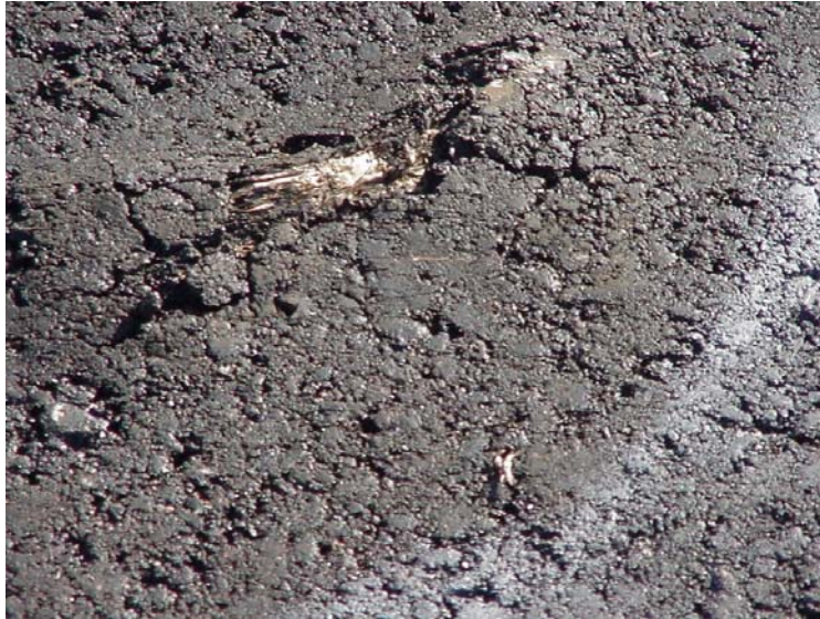
Figure 8 - Contamination of HMA with wood chips.
