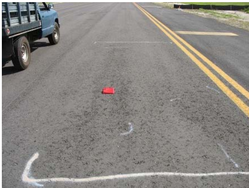
Figure 5. Surface of Pavement showing Segregation.
