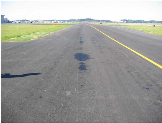
Figure 9. Water flowing out the surface of a pavement.
