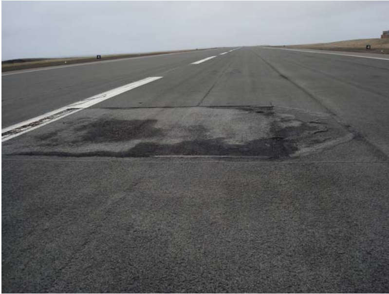
Figure 4. Patching that exists on the 31 year old pavement.
