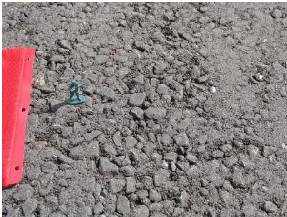
Figure 6 - Close-up of Segregated area showing porous surface.
