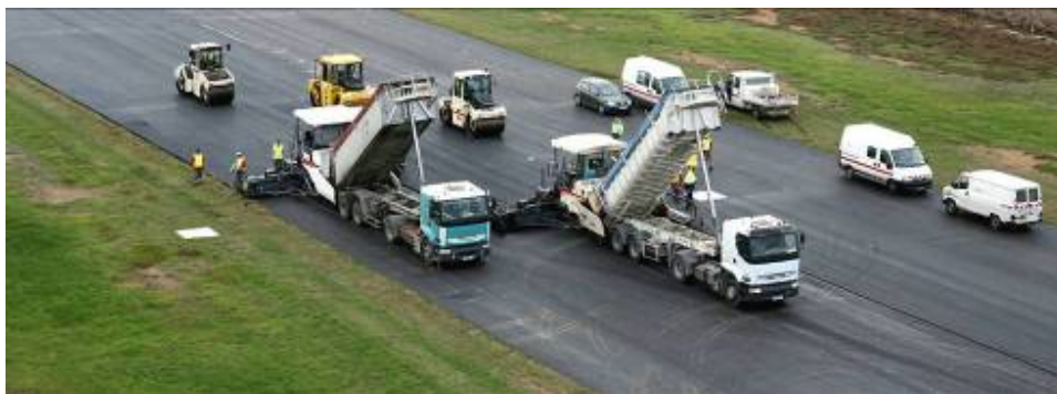
EBT: application of 4500 tons of warm mix asphalt BBA 0/10, aerodrome of Candillargues (photo credit: EIFFAGE company Public Works)
