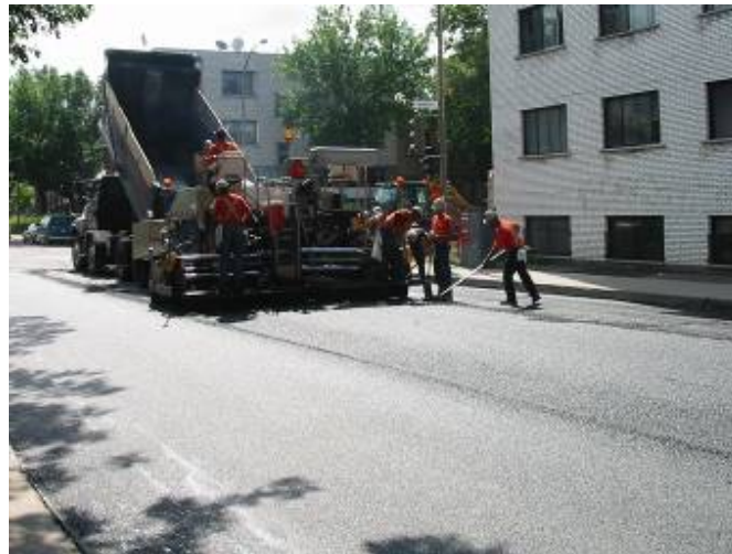
Application of warm-mix asphalt to aspha-min ESG-10 PG 70-28, Bali Street in Montreal (Canada), August 2005 (photo credit: Y. Paquin DJL - EUROVIA)
