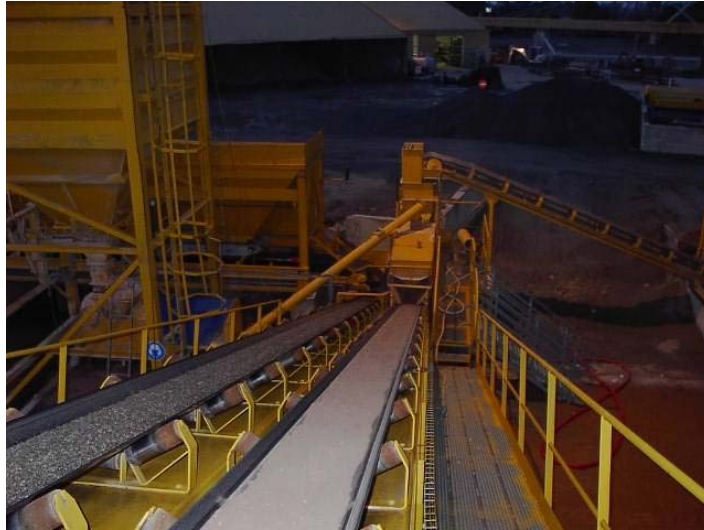
Figure 6 – Cold mix plant with double conveyor
