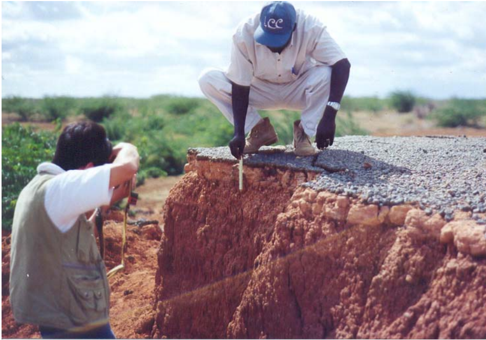
Fig. 22 El Nino Damaged Tana Basin Road Project
