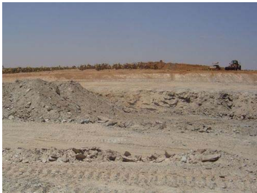
Figure 2. Use of very dry mica schists on a motorway works site in the Marrakech area (Morocco).
