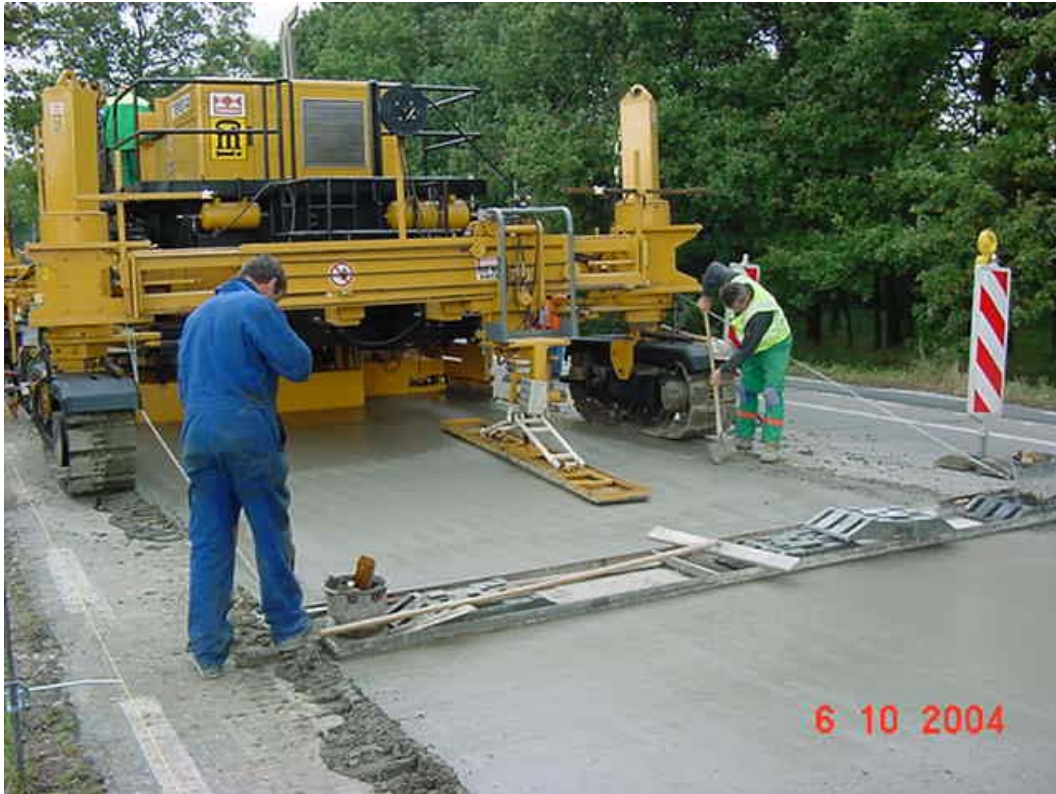
Figure 3 - Finishing stage, prior to the application of a curing compound or covering with plastic sheet
