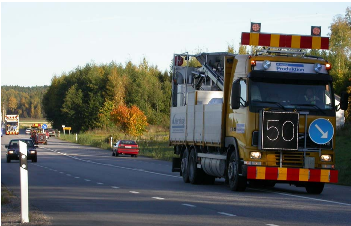
Figure 10 - LED (digital) signs mounted on trucks displaying the recommended speed during road marking operations. Enköping, 50 km northwest of Stockholm, 2005. Observe the white radar equipment (type SR3+) down to the right of the truck.
