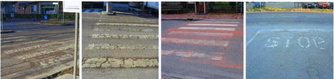
Figure 17 – Road markings in poor maintenance condition
