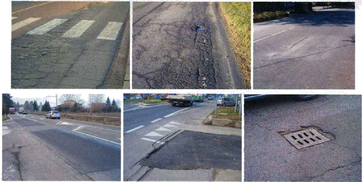
Figure 18 – Poor maintenance conditions of road pavements
