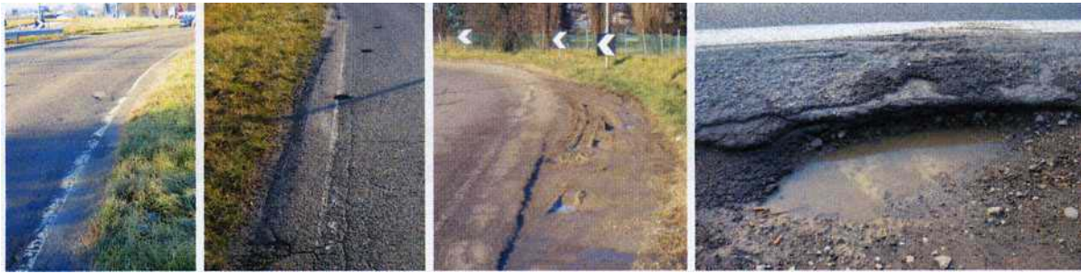
Figure 4 – Narrow and unpaved shoulders
