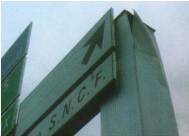
Storm of January 1998 (Photo J. Berthelémy)
