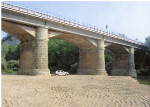
Photo n° 22 – General sight of the bridge on the river Bormida, along the ex-state roa 30, at Terzo d’Acqui
