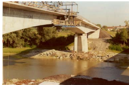
Photo n° 13 – Beam concave of the new bridge on the Tanaro along the main road 77
