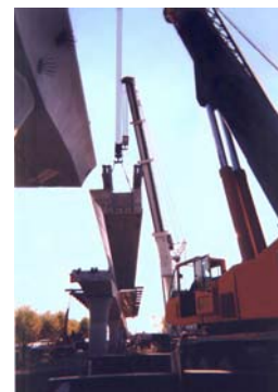
Photo n° 10 – The new viaduct along the main road 87 – Launching of the viaduct last span
