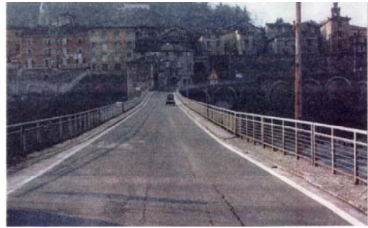
Photo n° 27 – Sight of the “original” road system of the bridge on the Scriva, along the main road 143
