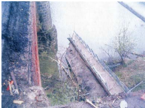
Photo n° 24 – Collapse of the first beam – mountain side of the bridge along the ex-State Road n° 30 at Terzo, near Acqui Terme.
