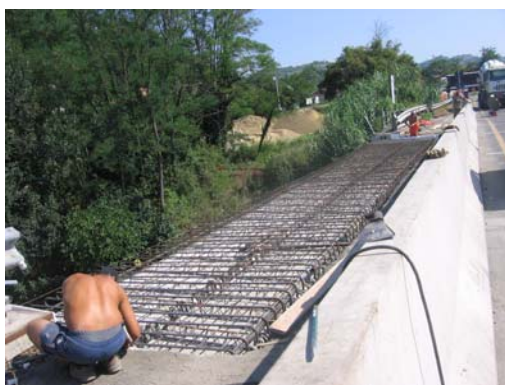
Photo n° 25 – Iron bars placed on the new reinforced concrete slab near the first restored span of the bridge of Terzo, along the ex-State Road n° 30
