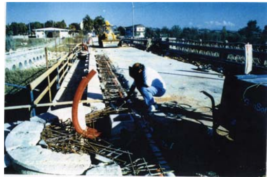
Photo n° 7 – The bridge along the main road 85 “Castelnuovo Scrivia – Alluvioni Cambiò” at Castelnuovo Scrivia – The restoration works of the road system.
