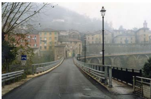
Photo n° 4 – The bridge along the main road 143 “Serravalle – Vignole”, when the works were finished
