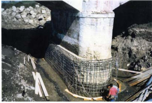
Photo n° 11 – Plinths and piers reinforcement of the bridge along the main road 85 “Castelnuovo Scrivia – Alluvioni Cambiò”
