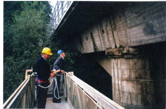
Photo n° 23 – Degradation condition of the bridge along the ex-state road 30 at Terzo, at the beginning of 2000
