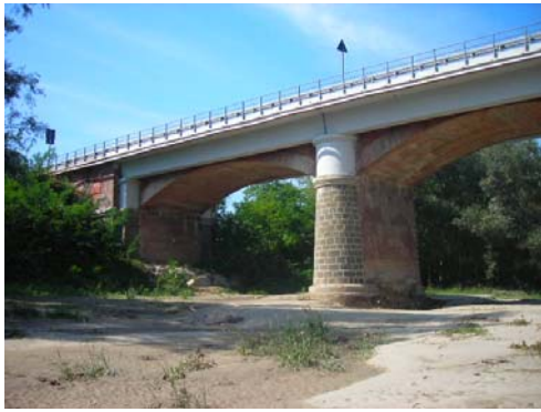
Photo n° 26 – Sight of the bridge of Terzo, along the ex-State Road n° 30, when the works were finished
