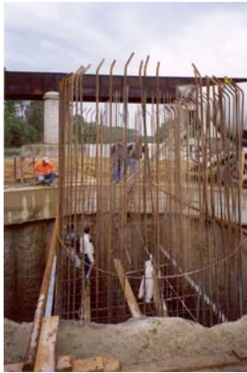
Photo n° 16 – Foundations “at well” of the piers of the new bridge along the main road 77
