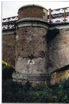
Photo n° 6 – The bridge along the main road 85 “Castelnuovo Scrivia – Alluvioni Cambiò” at Castelnuovo Scrivia, damaged by the torrent Scrivia flows.
