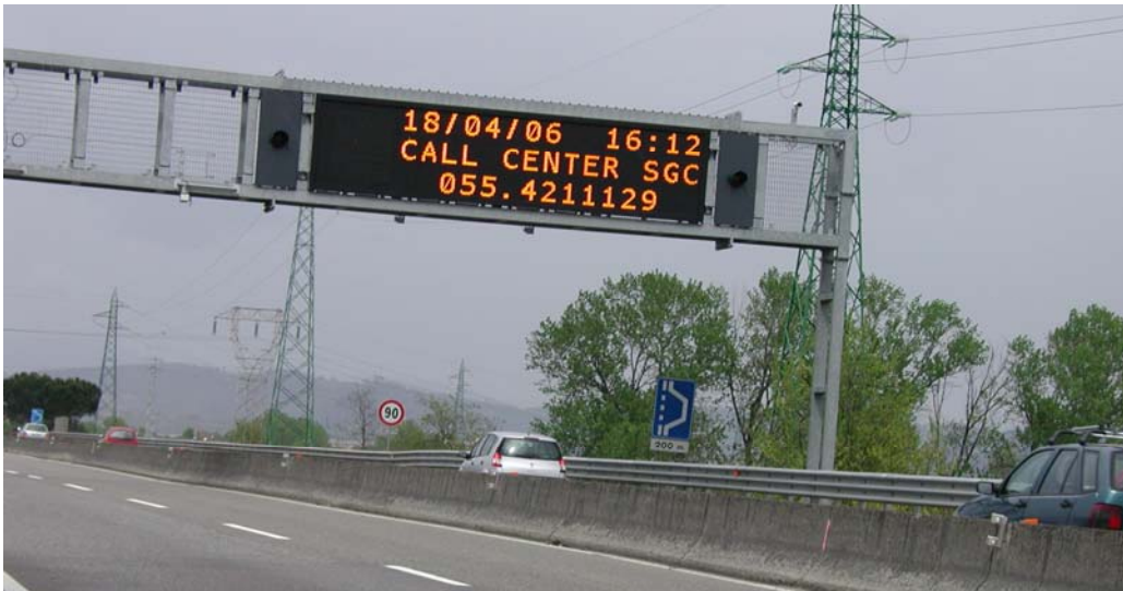
“Figure 6 - Variable messages panels located along the infrastructure”
