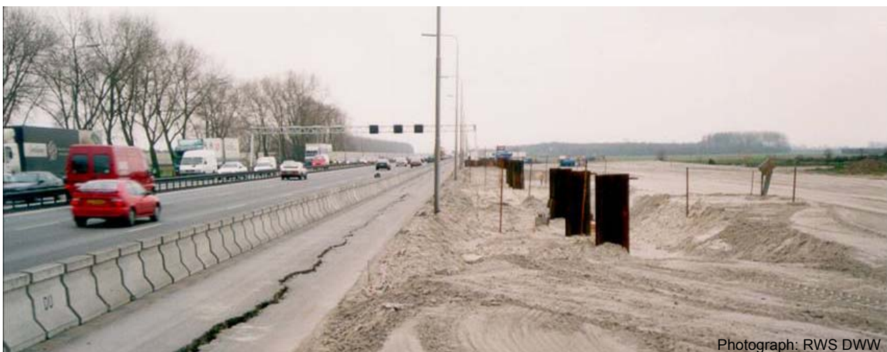
Figure 2 - Pavement cracking at road widening project
