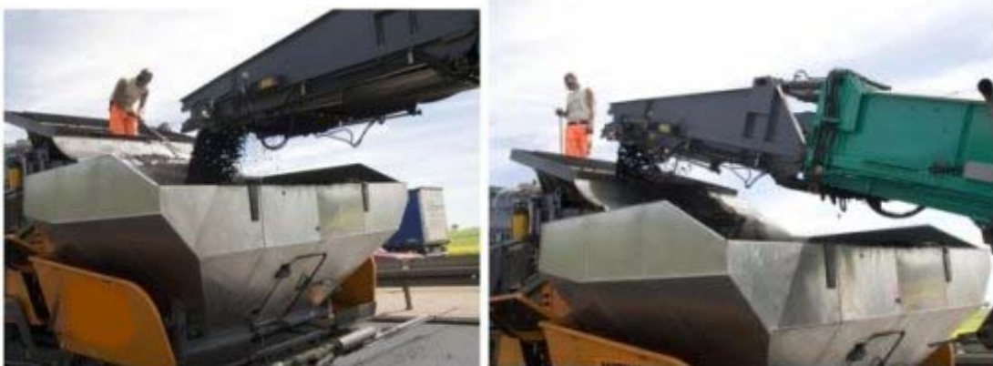
Figure 7 The binder finisher is being charged: binder on the left and surfacing on the right.
