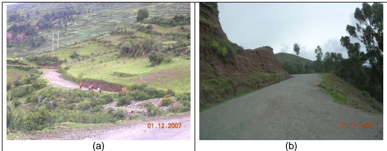
Figure 2. Example of Micro-enterprise work on Rural Roads in the Province of Cusco.
