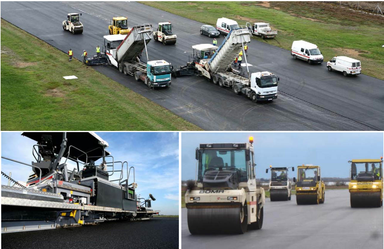
Figure 9. Example of a 3100-ton LEA ® roadwork for an aerodrome near Béziers (France).
