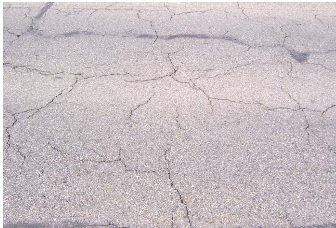
Figure 8: fissuration du support
