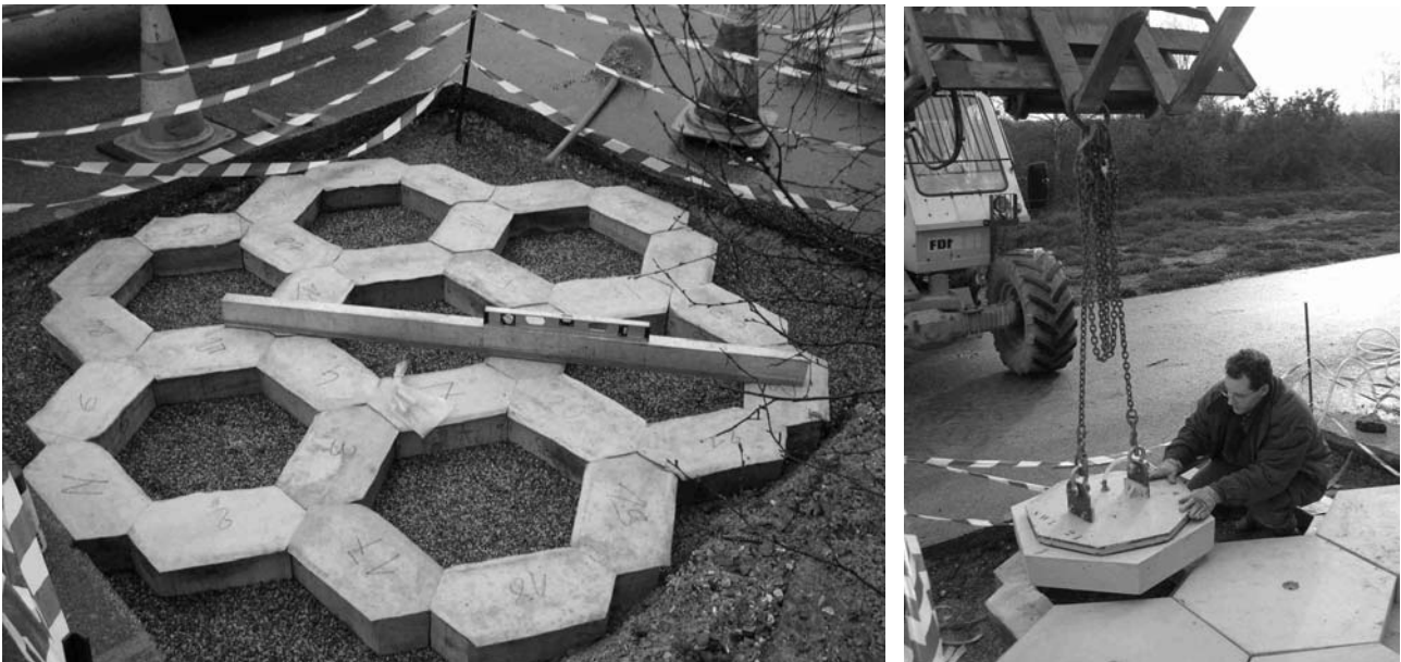
Figure 6 - The Rouen solution: wood beams covered with a geotextile sheet on which concrete slabs are positioned. The beams can be applied manually owing to their light weight.
