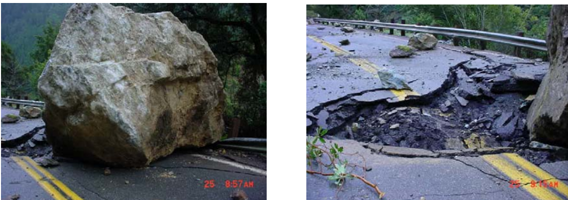
Figure 3 - Photo of Land Slide, February 2007 - Humboldt County, CA, State Highway 96.
