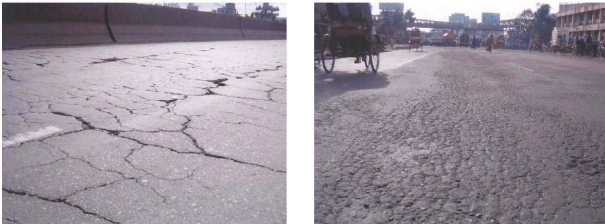
Figure 4: Fatigue cracking observed in Dhaka-Chittagong road (N1) (chainage 0-9 km) [8]
