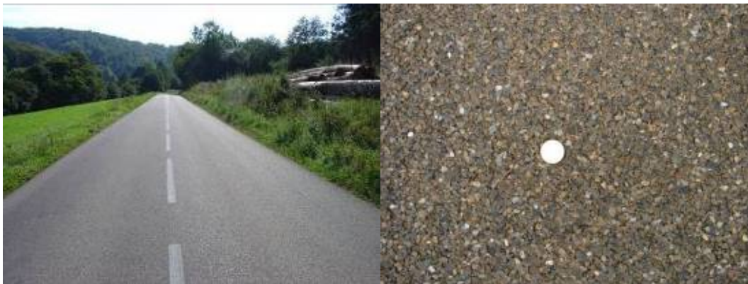
Photo 12 – view of the pavement after 30 months
