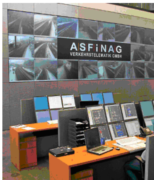
Figure 7 – Inside view of TMIC
