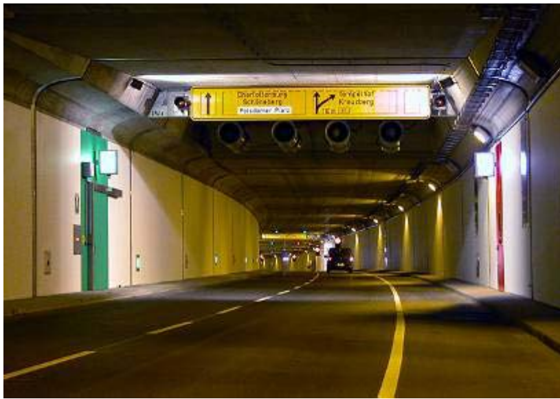
Figure 12 - Tunnel safety equipment in the Tiergarten Tunnel in Berlin
