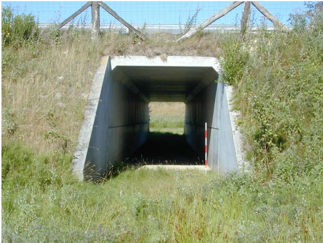
Figure 7 - Dry underpass with the closest entrance opening into an artificial depression as the road surface of the motor way is constructed in level with the surroundings.
