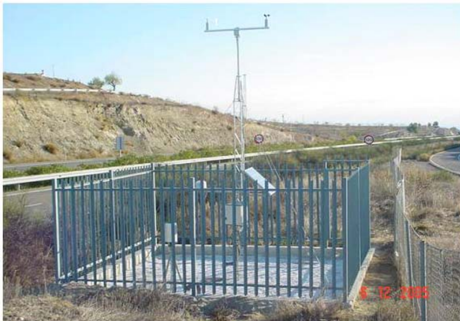
Figure 7- Weather station at Lorca for winter maintenance management purposes
