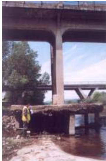
Figure 7 - Foundation with deep scour
