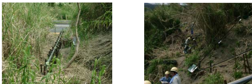
Photo 2 - Installation example of sensor for slope failure measurement
