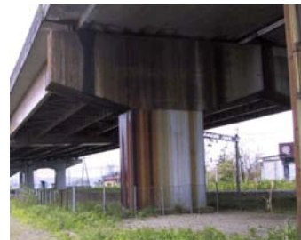
(b) No damage with pier retrofit (2004 Niigata-ken Chuetsu Earthquake)
