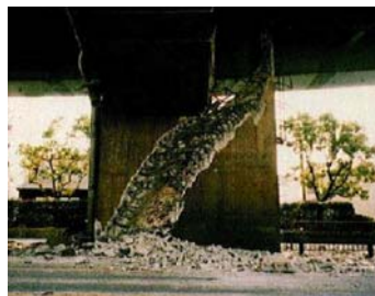
(a) Bridge pier damaged by the 1995 Hyogo-ken Nanbu Earthquake
