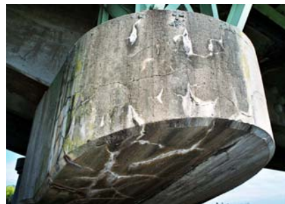
Photo 3. Deterioration due to an alkali-aggregate reaction
