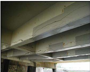
Photo 1. Deterioration due to chloride attack
