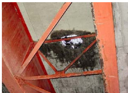
Photo 2. Decay of floor board due to fatigue
