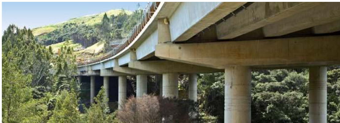
Figure 4 - Partly completed eco-viaduct shows the small footprint created during construction to retain existing ecosystem beneath the structure
