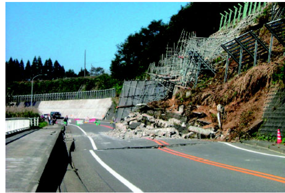
Photo 3 Slope collapsed at Ushigashima, national highway Route 17 [1]
