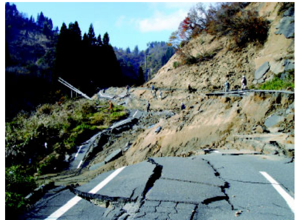
Photo 6 Collapsed road at Higashi-Takezawa, national highway Route 291 [1]
