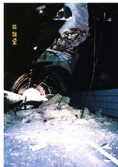
Photo 2 Damage inside the Wanazu Tunnel, national highway Route 17
