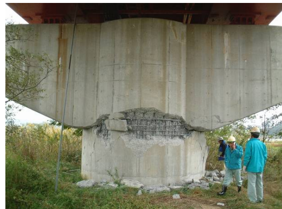
Photo 5 Damaged bridge pier of the Ojiya Bridge, national highway Route 17 [3]
