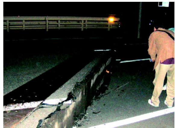
Photo 1 Road level difference at the Mitsuke Bridge, national highway Route 8 [1]
