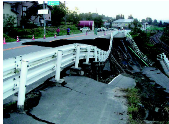
Photo 4 Collapsed road at Tenno, national highway Route 17 [1]
