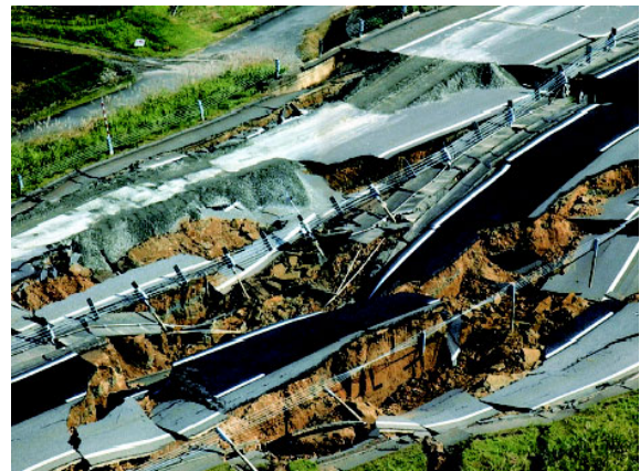
Photo 7 Damage to Kan-etsu Expressway (between Horinouchi IC and Echigo-Kawaguchi IC) [1]
