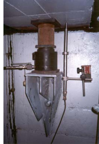
Hydraulic racket between steel bracket and concrete beam
