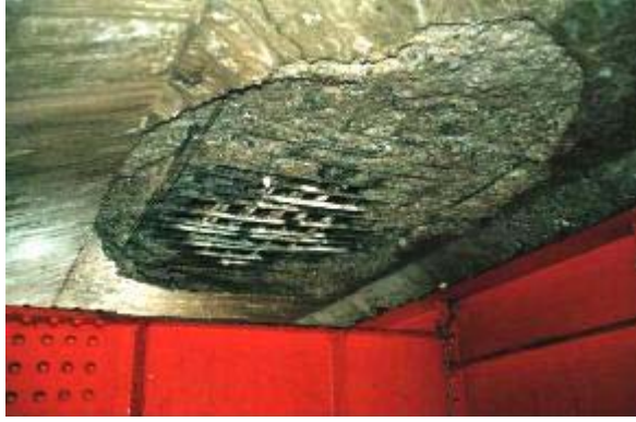
Photo 2 - Dropping off of concrete of RC Slab
