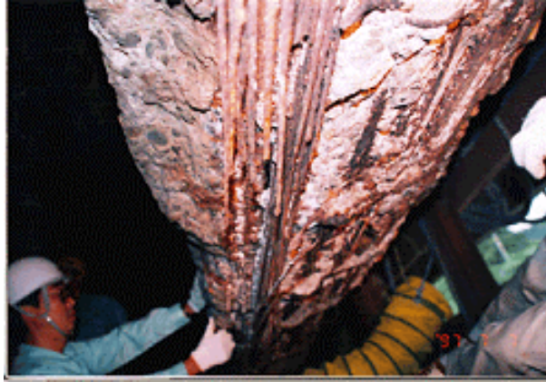
Photo 3 - Chloride damage of PC girder
