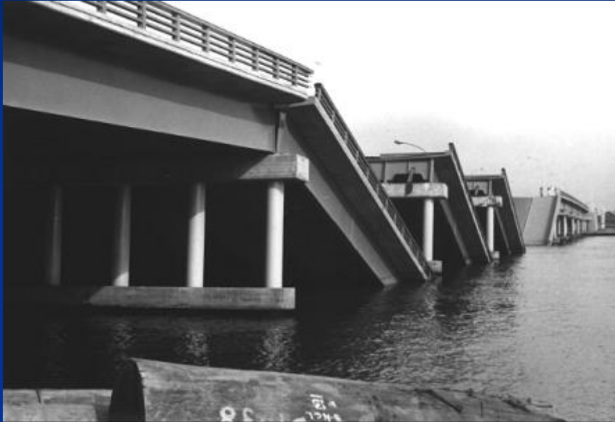
Falling Down of Superstructure by Niigata Earthquake (1964, M7.5)
