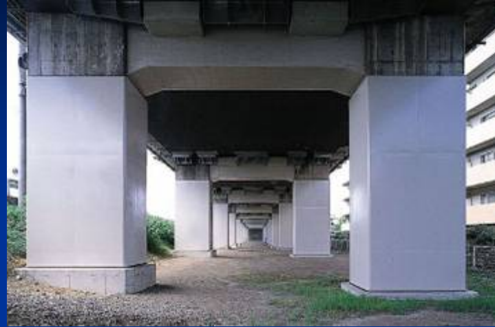
Strengthening of RC piers by RC, steel plate, or carbon fiber sheet
