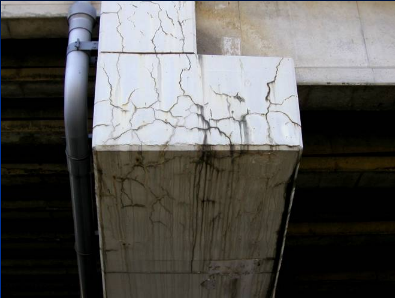
Damage due to Alkali Silica Reaction
