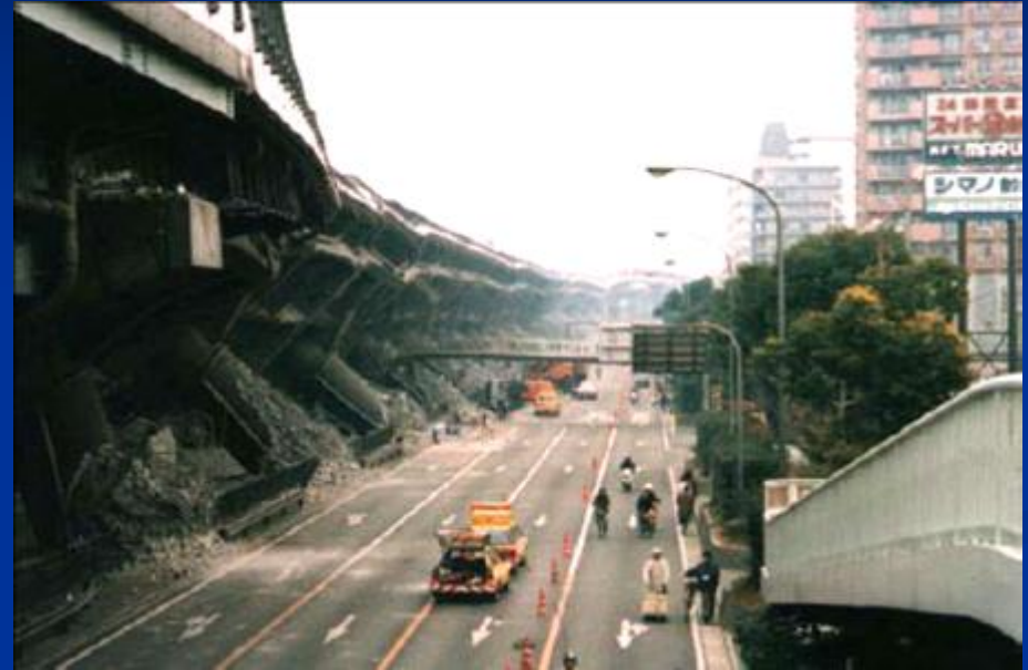
Collapse of Substructure by Kobe Earthquake (1995, M7.3)
