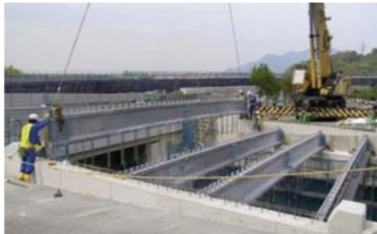
Photo 5: Montage des poutres en BFUP Photo 5: State of erection of UFC girder
